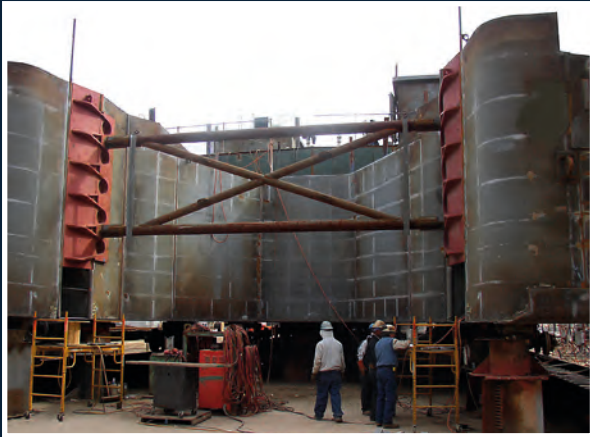
Socket plate installation to the barge in progress. The assembly jig (not included in Beacon's scope of supply) between the red socket plates ensures correct spacing.
