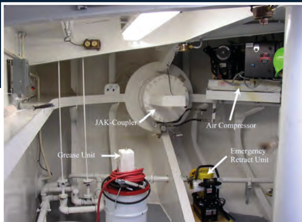
Couplers compartment in the bow of the pusher: the port side coupler unit assembly is clearly visible.
